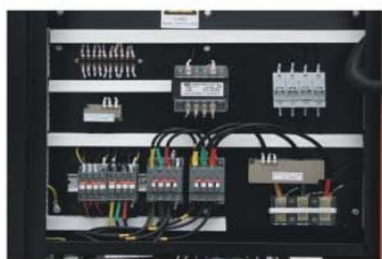
Electricity Board (Siemens/ABB PLC)
